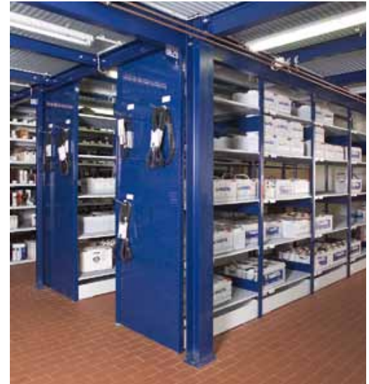
Battery storage on hazardous goods shelves with drip trays
